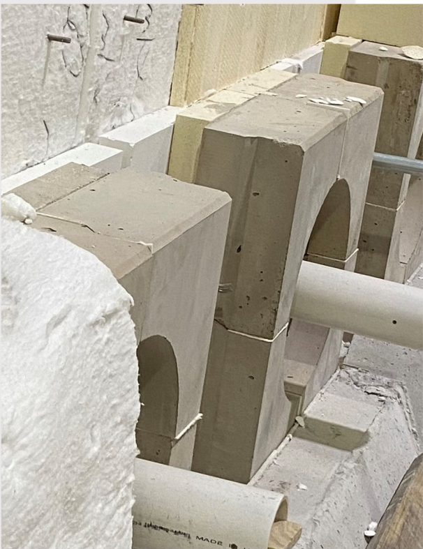
Insulation blanket, board, insulation brick, and Precast shapes installed around the rollers.
