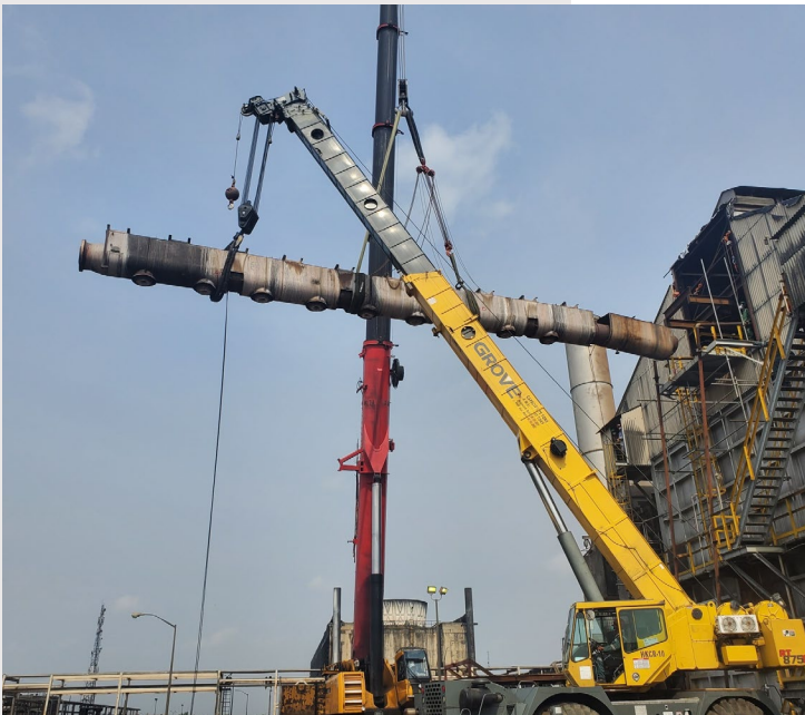
Tandem Cranes (220T + 60T) removing the OLD Transfer Line from the Penthouse in a single 80ft Long Piece
