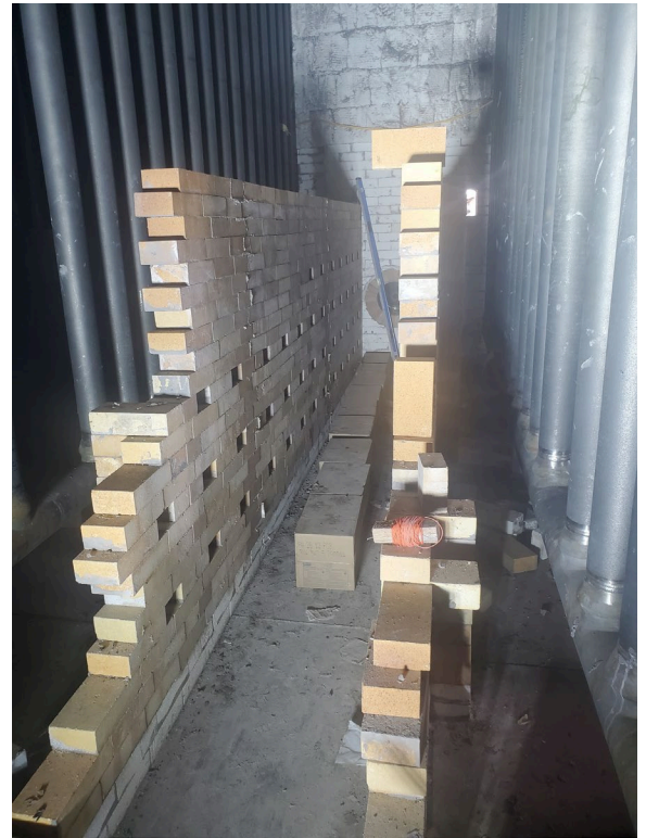
Tunnel wall inside Primary Reformer in construction after NEW Harps were put in place.
