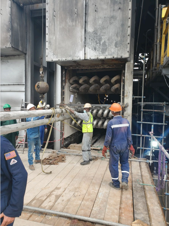
Tube Replacement ongoing at the Mixed Feed Coil. Crew used an Air Tugger to pull in new tubes sent from the US.
