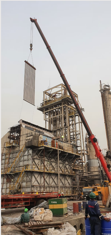
220T crane dropping in NEW Harp Assemblies (27) total from the Roof of the Penthouse.
