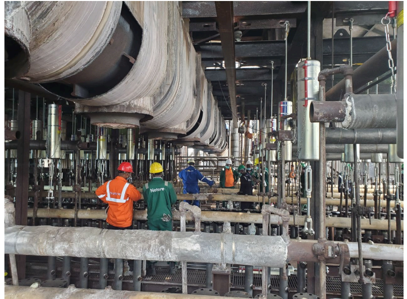
Penthouse view of the OLD Transfer Line and OLD Harp Assemblies below during the Demolition Phase.
